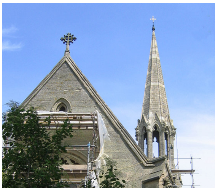
The repaired spire of Charlecote church has now emerged from the scaffolding that once surrounded it. The remaining scaffolding should all be removed by early in July
